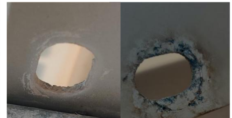
A picture of the rusty aluminum frame of the solar module from an offshore PV power station
